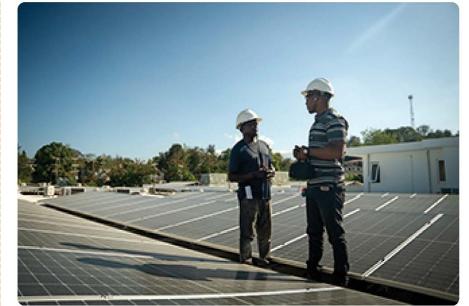
Members of the solar project team, Valdes Simon (left) and Smith Poucet (right), examine the panels on the roof of Hôpital Universitaire de Mirebalais. Photo by Mélissa Jeanty / PIH
